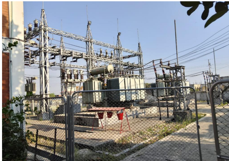
Figure 7-6: Substation Situated 6 km from Proposed Site
